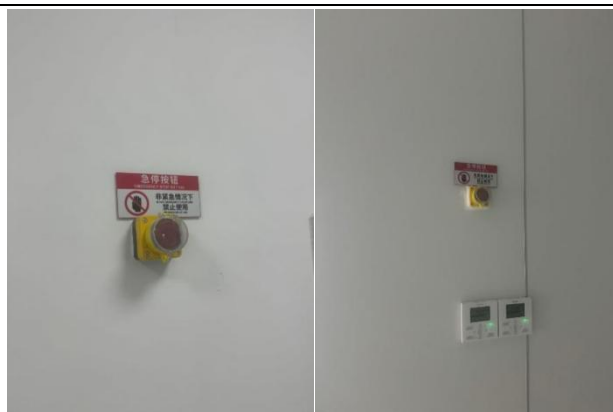
PET/CT 机房急停按钮
